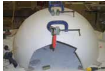
两组组成一个半球 Assembly of 2 quarter pieces to half a shell
